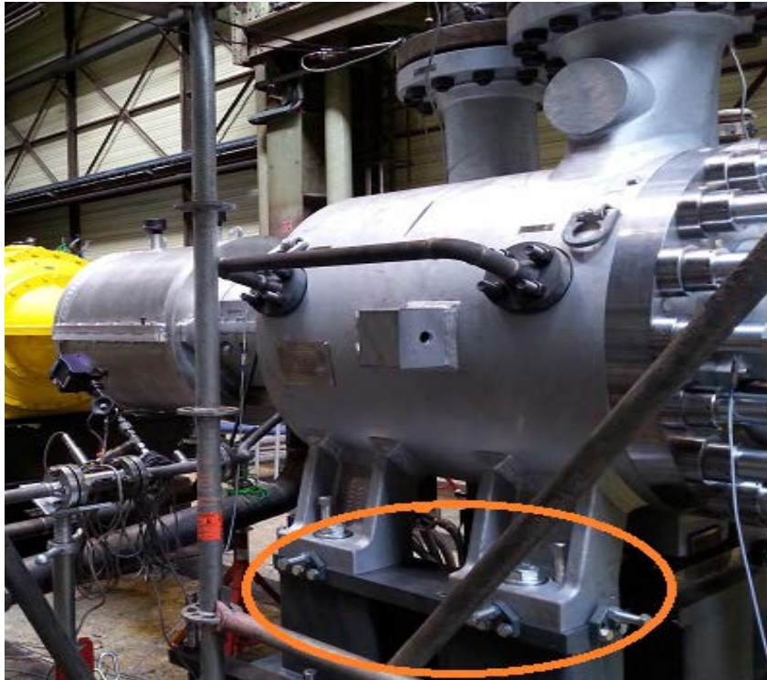
Fig 2 -Compressor MRT - Project specific base frame not used
